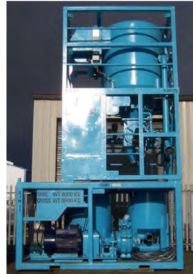
Assembled – Mixer and Surge Tank
